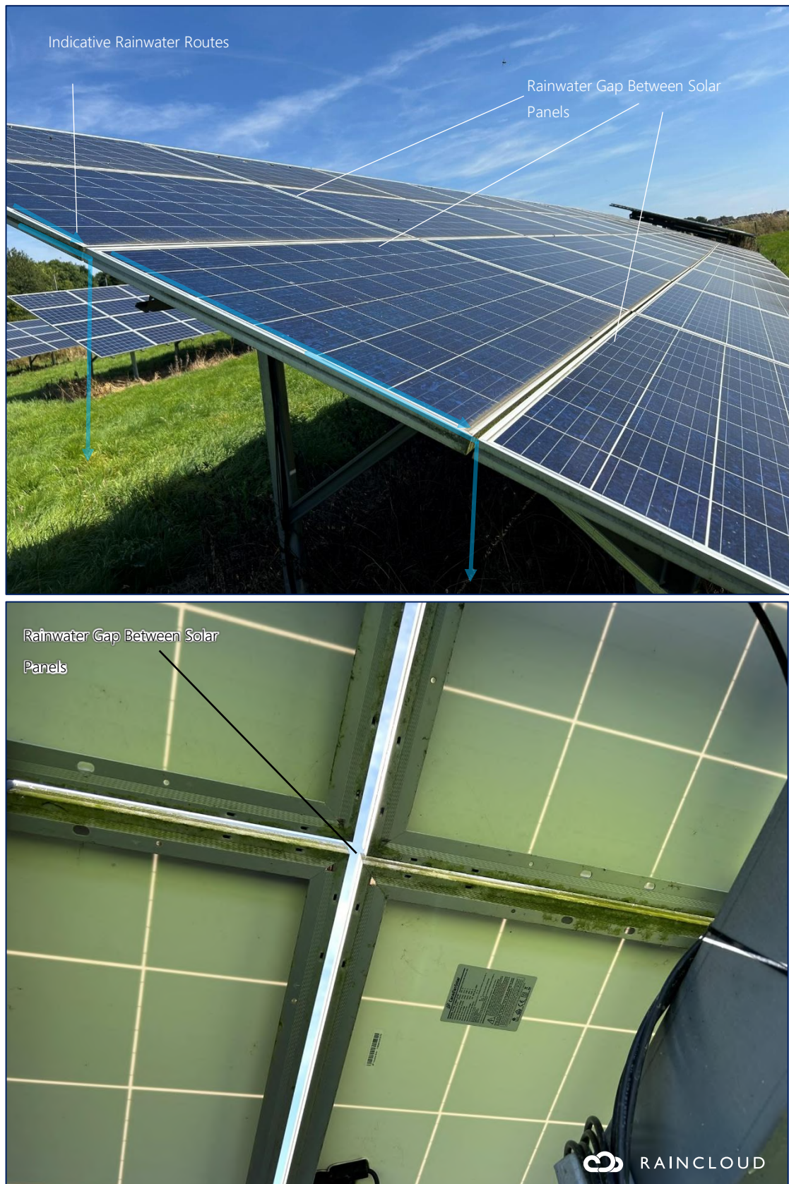
Plate 12-25 Rainwater gaps on PV array table
